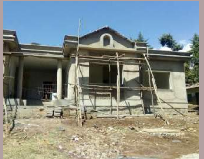
Ethiopia: Construction of new presbytery for the catholic community of Kochi of the Apostolic Vicariate of Nekempte
